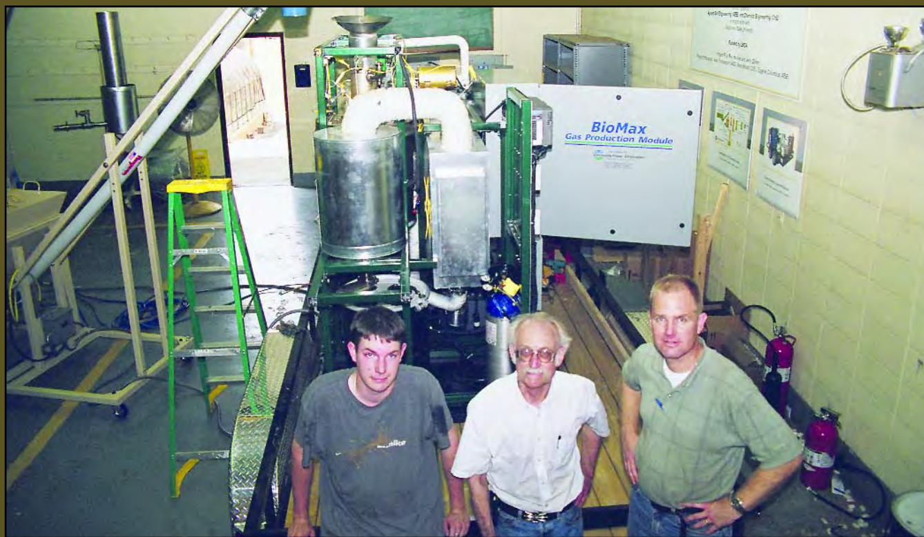
Community Power Corp. technicians Mike Walker, left, Jim Diebold and MAFES agricultural engineer Alex Thomasson during installation of the Biomax gasifier.
