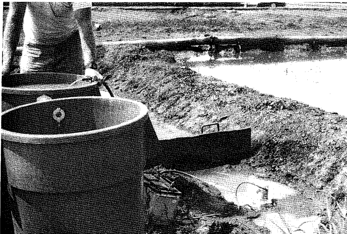
Figure 6. Measurements of seepage over time were obtained by pumping seepage water occurring in a 10-foot section of the levee into adjacent containers.
