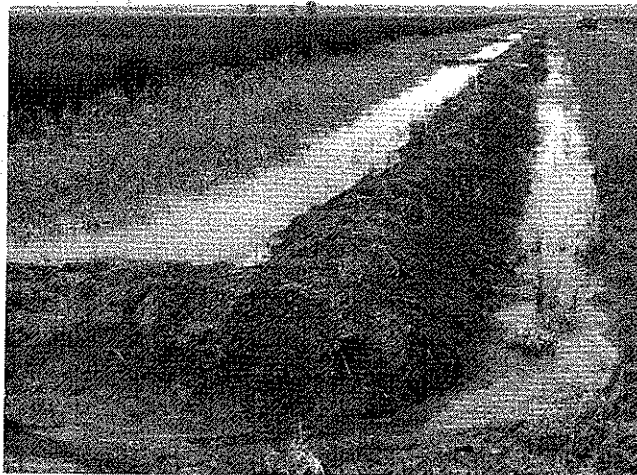
Figure 1. Example of seepage loss (right) occurring where a nonpermanent outside levee was constructed.
